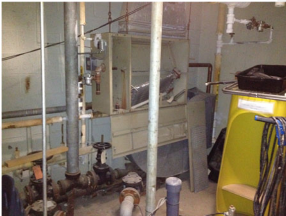
Storm shelter (south) in mechanical room
