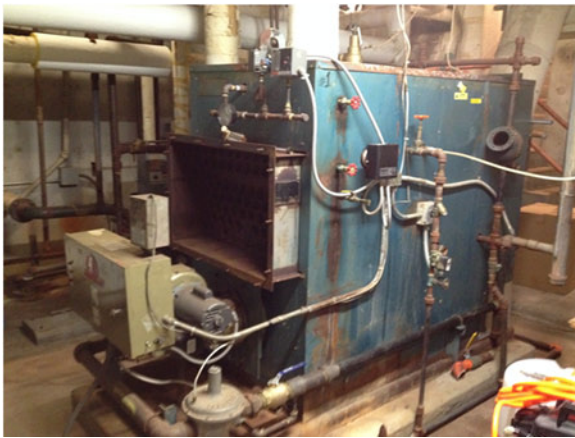
Boilers past useful life require replacement
