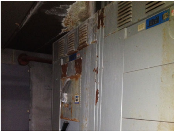
Water damage at building main electrical switch
