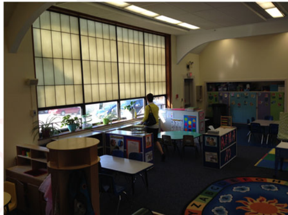
Kalwall window systems need to be replaced
