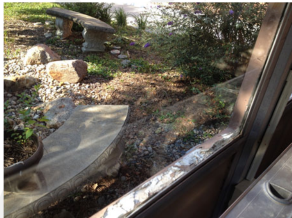
Single pane windows need to be replaced
