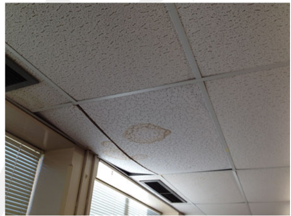
Ceiling tiles showing moisture & humidity damage
