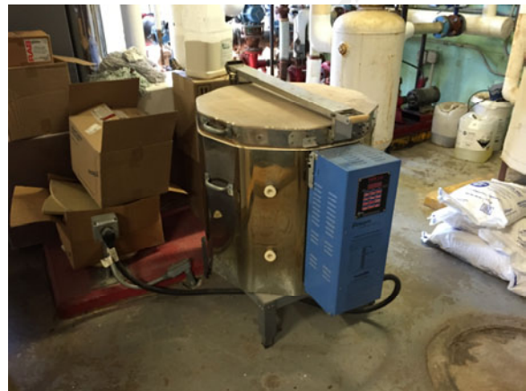
Kiln in boiler room (typical at most Elementary schools)
