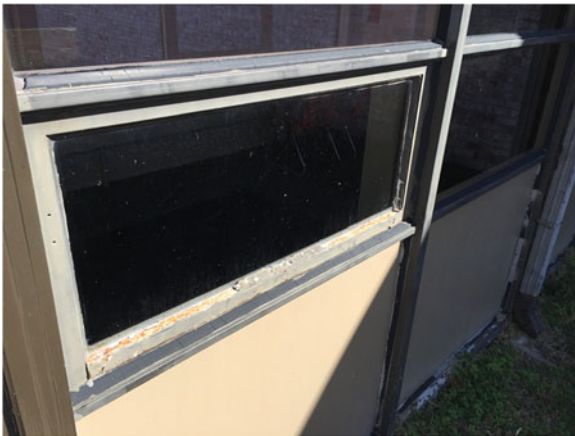
Single pane window needs to be replaced
