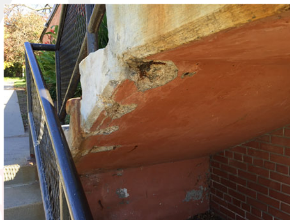
Deteriorated stair concrete needs repair
